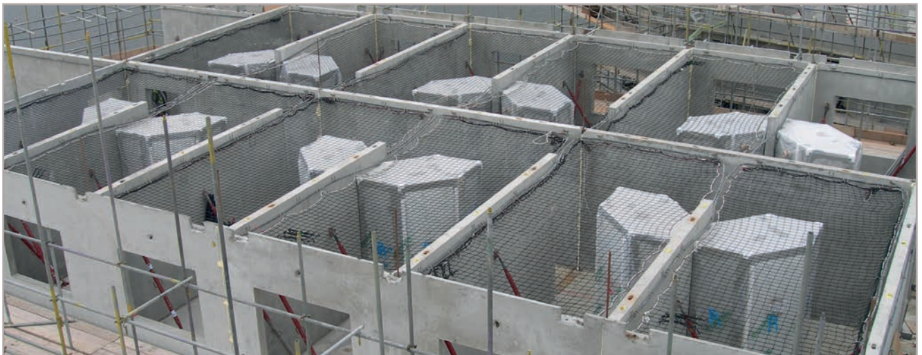
University of East London. Five seven-storey and four three-storey structures, creating 788 bedrooms, were erected within 33 weeks using crosswall construction.
