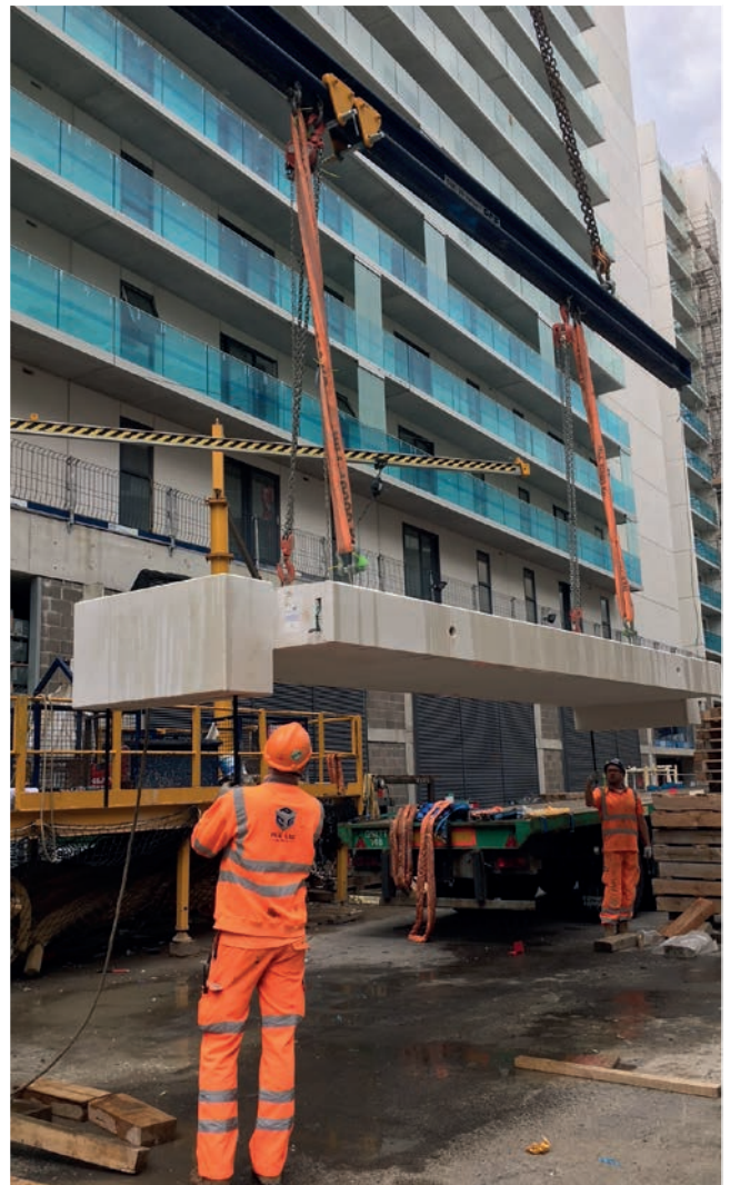
Chapel Wharf, Manchester, 995 apartments in four offsite-engineered hybrid constructed towers, up to 23 storeys. Image courtesy of PCE Ltd.
