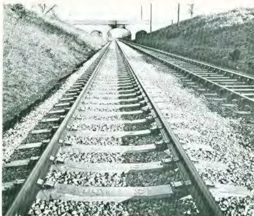
Prestressed sleepers improve the permanent way on British Rail's Western Region—where long welded rails are installed.
