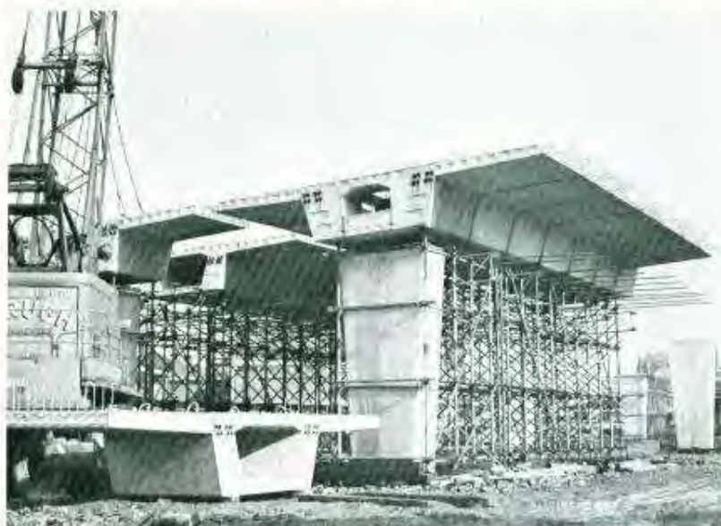
25-ton precast prestressed deck sections of Mancunian Way elevated road. Consulting engineers: G. Maunsell and Partners.
