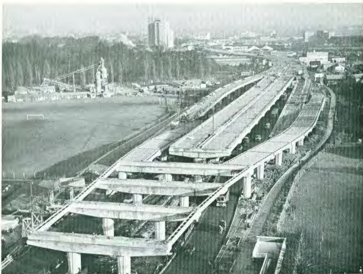
Prestressed standard bridge beams were used for the deck of the elevated section of M4 motorway. Consulting engineers: Sir Alexander Gibb and Partners.
