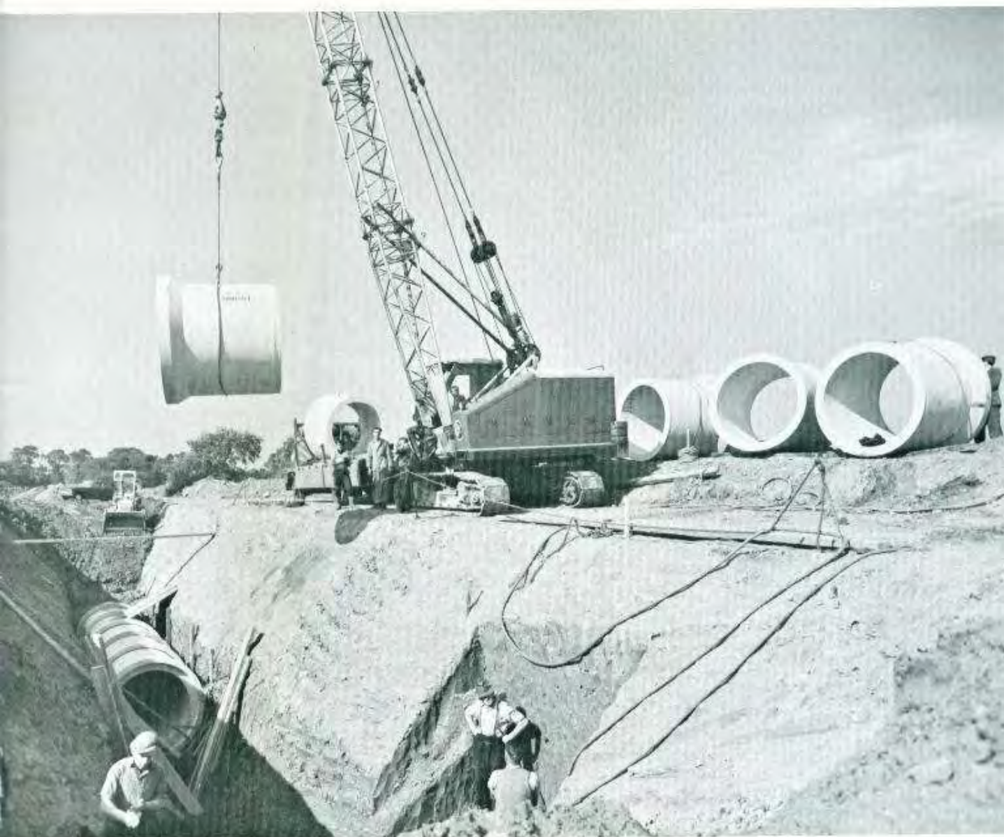
Extra-strength, flexibly jointed precast pipes—63 in. diameter —being laid at Widnes, Lancs.
