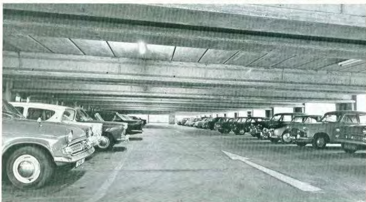
Below: Long-span prestressed T beams provide the uncluttered floor areas for Croydon's multi-storey car park. Consulting architect: D. H. Beatty-Pownall, FRIBA.
