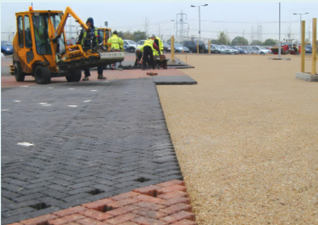
Machine laying of concrete paving units offers a particularly efficient solution for permeable as well as conventional block paving.
