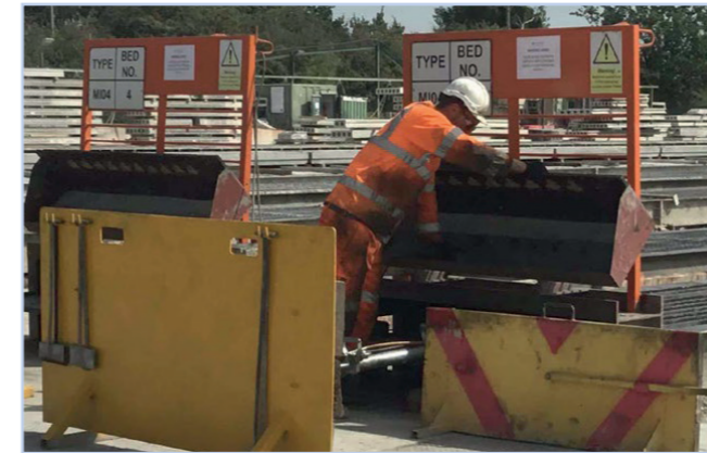
Figure 7.20 Sliding guard covering stressed wires.
